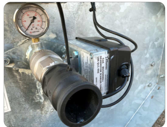
Automatic shut-off using electrical valve
